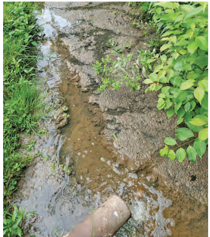
The effluent sample had E. coli levels more than 192 times the facility’s permitted limit, posing a threat to the community whose drinking water well was located near the stream.
